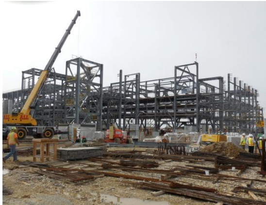
Iowa Fertilizer Company Area 10 Buildings 002, 007, 010 – Wever, IA Client: Tapia/Beck Steel – Ongoing structural steel connection design project for a Fast-Track ammonia processing plant expansion. The total tonnage without connecting material is estimated at 1,600-Tons.
