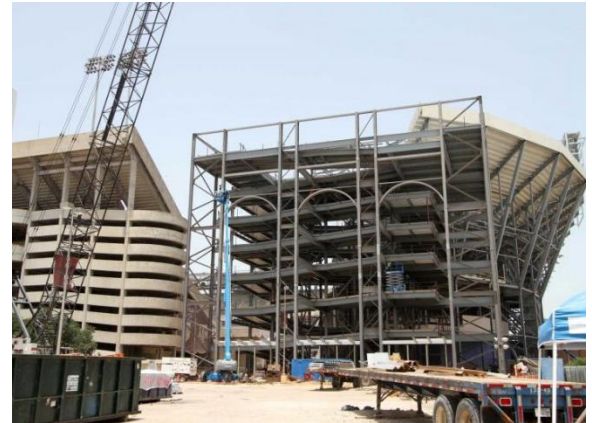
Texas A&M Kyle Field – College Station, TX Client: Beck Steel – Ongoing design assist and constructability review for all stairs and railings for the renovation of stadium. Over 20 individual stair and railing systems are being modified and installed.
