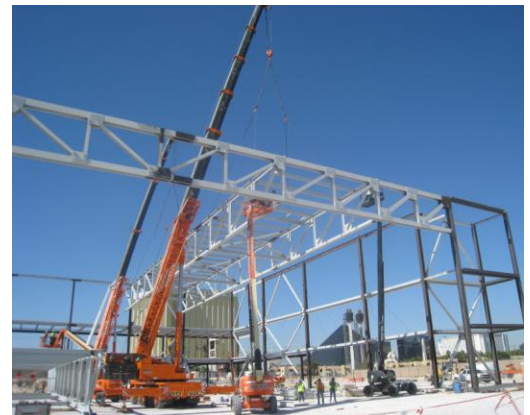
Sands Aviation Hangar – Las Vegas, NV Client: Union Erectors – Designed rigging and developed an engineered erection plan for the construction of a new private hangar for the Las Vegas Sands Corporation at McCarran International Airport.
